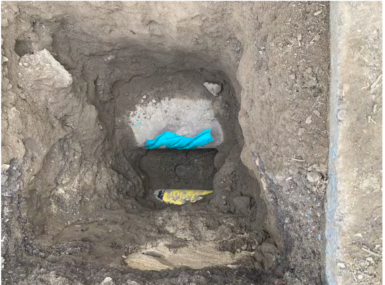
Photograph 6: Daylit, southernmost, active 16-inch Kinder Morgan pipeline (top in blue) and unknown line (bottom in yellow). Coating of 16-inch pipeline repaired (blue). Top of active pipeline 3.5 feet below ground surface. Depicted excavation extends 7 feet deep and 4 feet by 4 feet in length, looking south.
