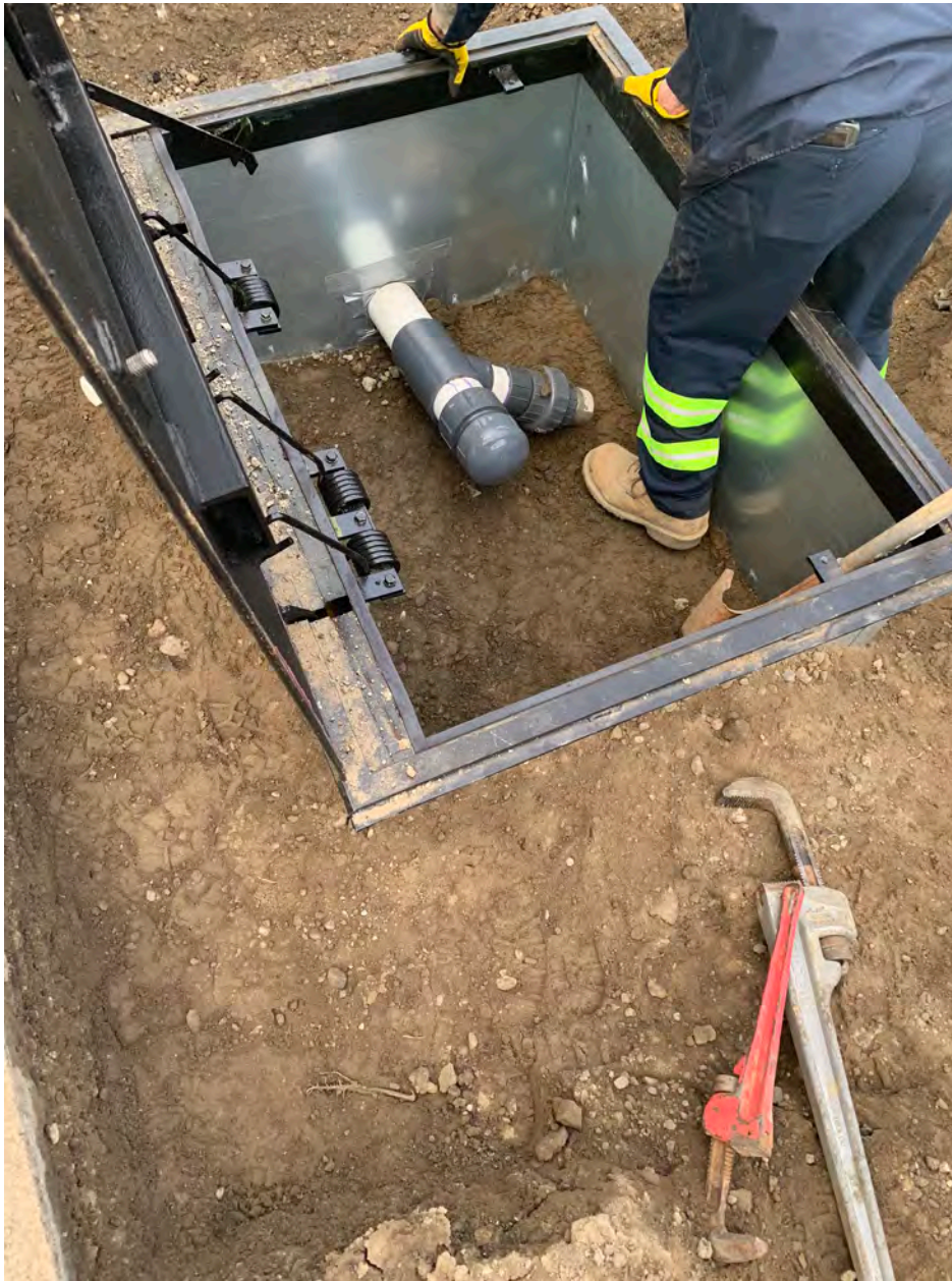
Photograph 8: View of BS-03 well vault installation and stub-out, looking west.
