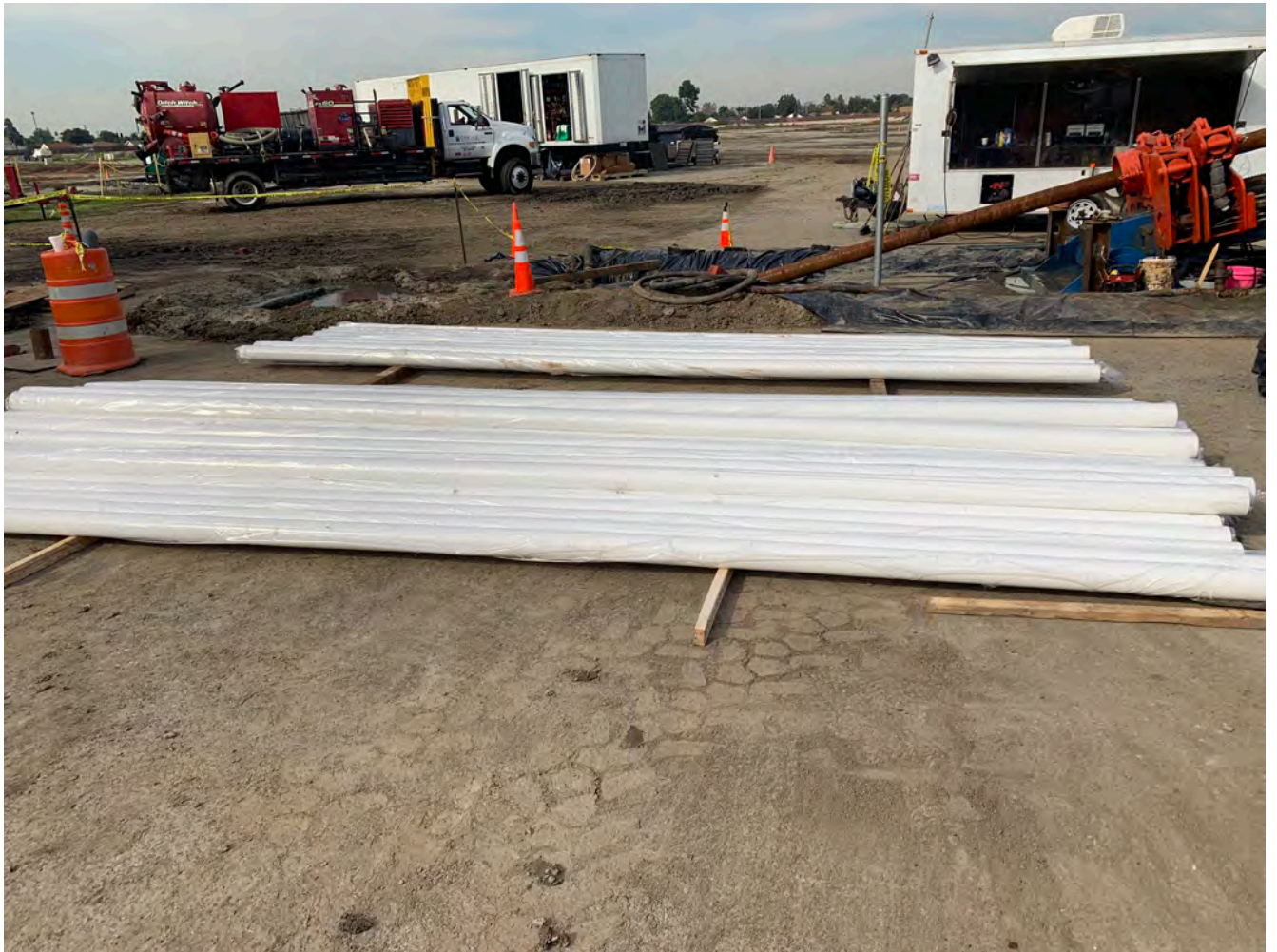
Photograph 4: View of 4-inch-diameter PVC well screen and blank casing for BS-03, looking southwest.
